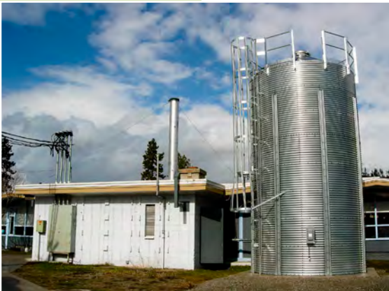
Wood pellet silo and boiler room at Troy School
